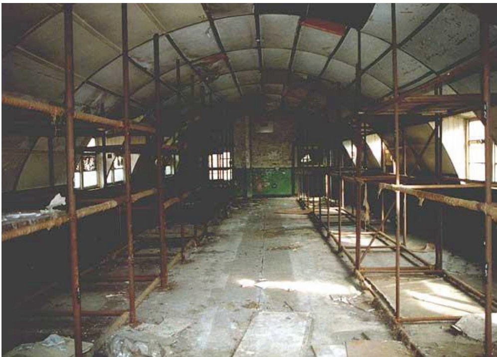
Interior shot of one of the office buildings on the operations site. During wartime this building would have been laid out with desks, typewriters, telephones, and bustling with administrative personnel. Post war, this building and many others like it were used to provide temporary accommodation to many Polish servicemen, who on release from POW camps did not wish to return to their homeland.
