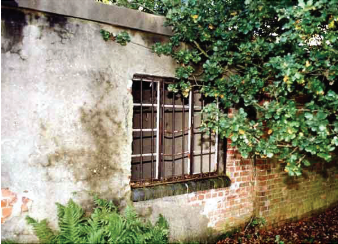
Iron bars protecting the windows clearly indicate the importance of this building. It was in fact the Norden bombsite store.
