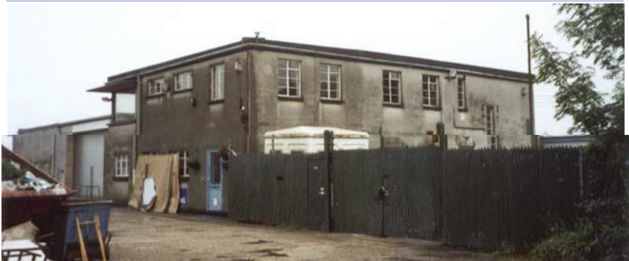
Rear view, it is only from the back that the original building can be identified, the three top floor windows on the right side and the long thin window on the far right (the 8ft high staircase window) show the original buildings dimensions. The two windows on the left side are in the new extended section 2002 (© Robert Truman)
