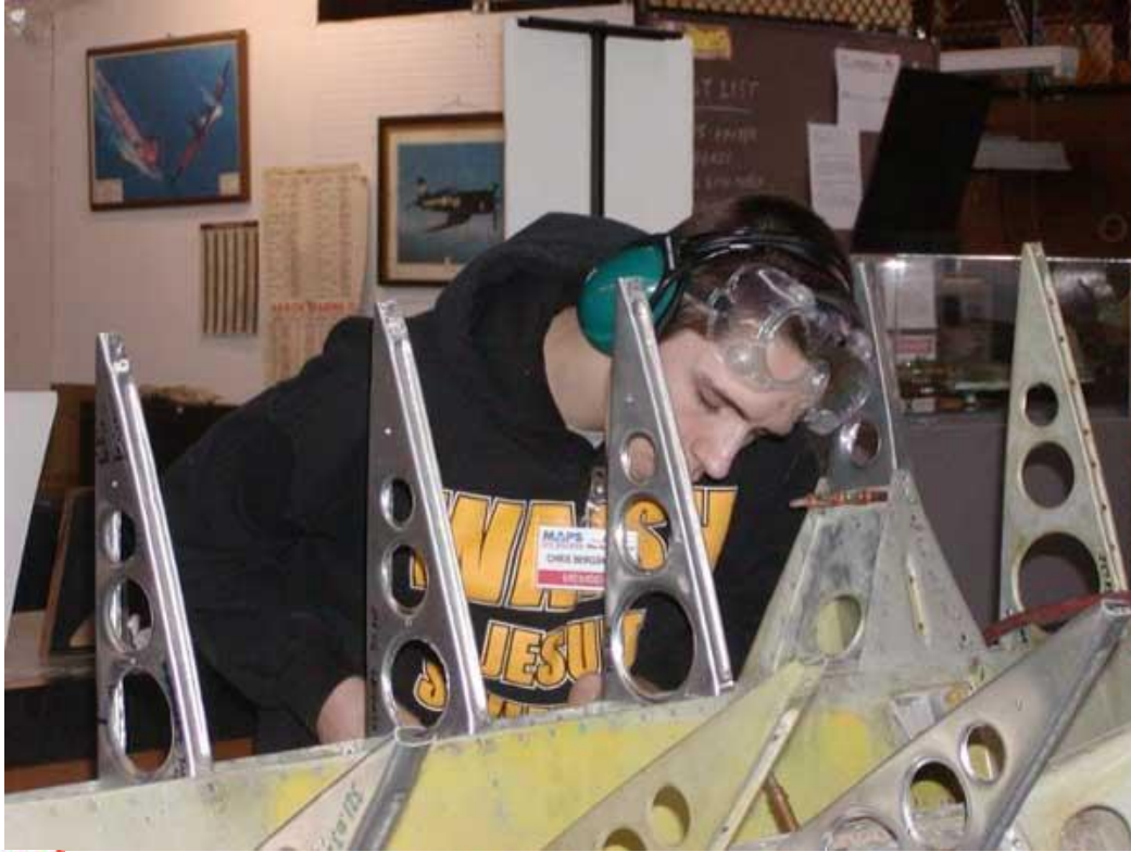
NEW! working on attaching the new ribs back on the B-26 aileron ♦ Photo ♦ Rick Willamon
